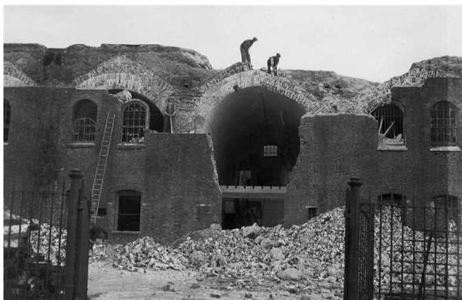
Fort Pitt Hospital was demolished in part to make way for the Girls School
