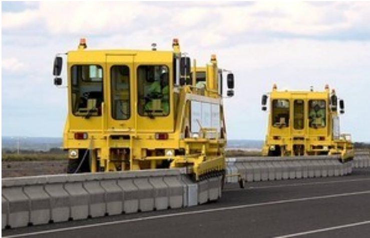
Two Barrier Transfer Machines in action, each moving the barrier one lane's width
